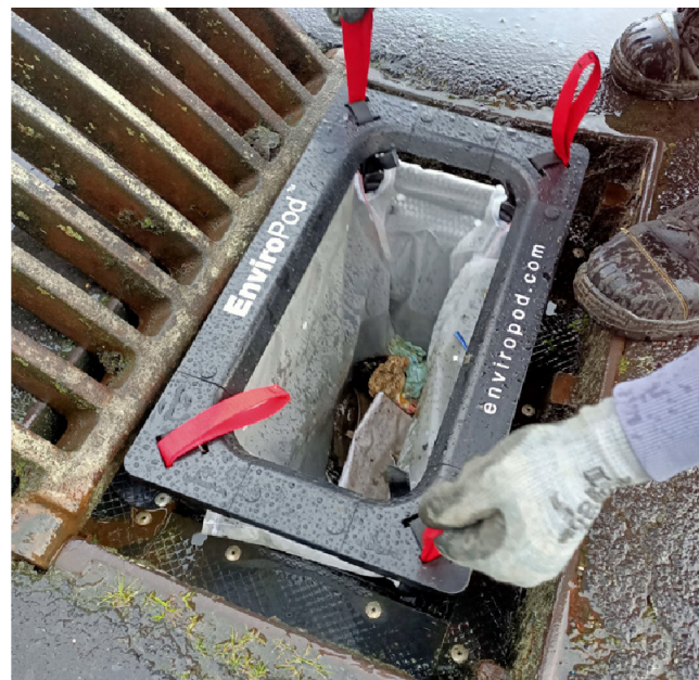
Figure 4: LittaTrap™ seen with 1mm liner installed to target micro-plastics such as plastic pellets. Hand maintenance shown.
