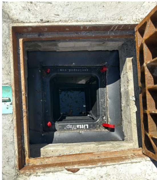
Figure 7. The EnviroBasin screening basket installed in the catch basin, accessible from the surface for inspection and litter removal.
