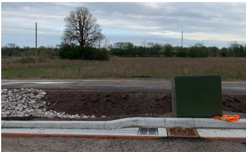
Figure 3. The installed EnviroBasin (right) with the trench drain running along the curb (foreground), which collects catchment runoff and forms the influent sampling point.
